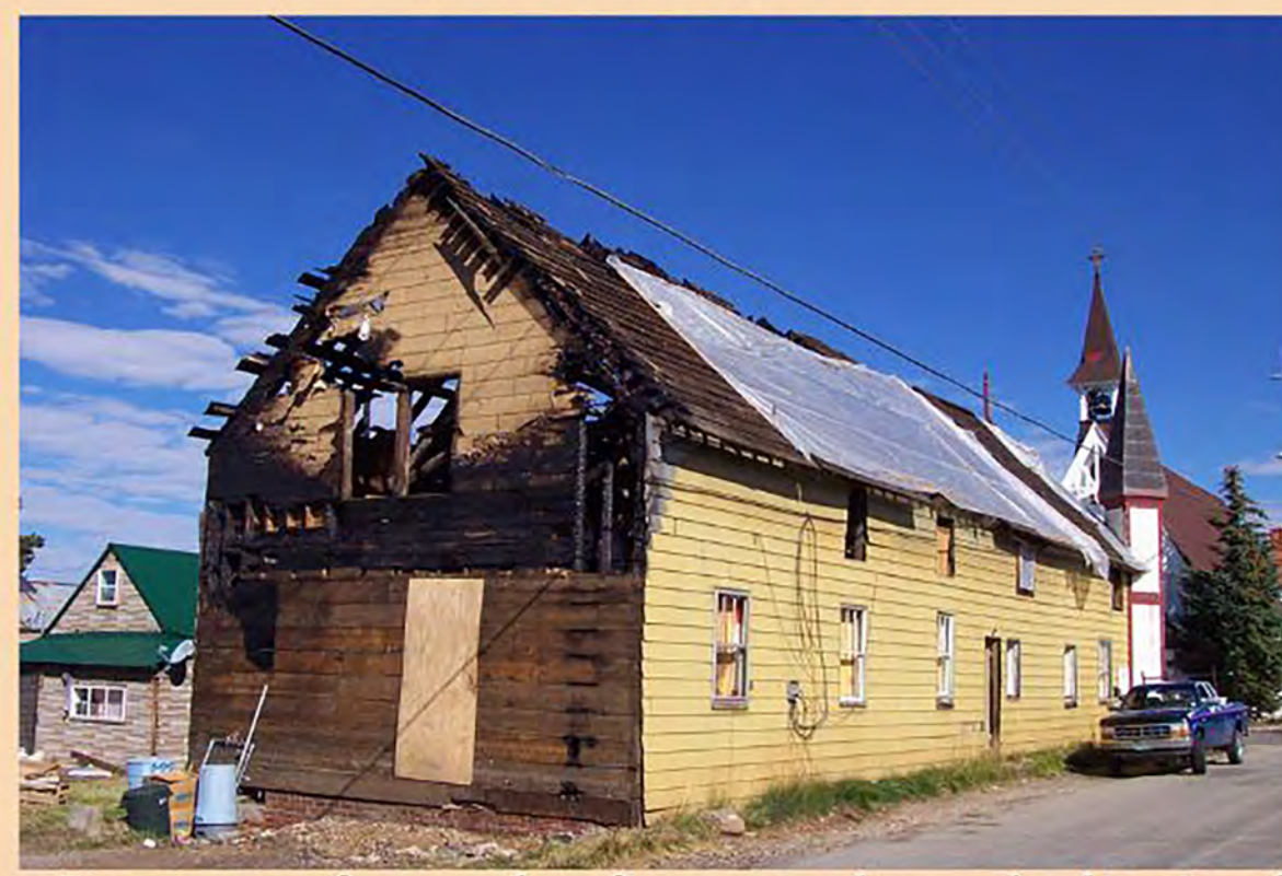
Damage from the fire was largely limited to the southern end of the building
